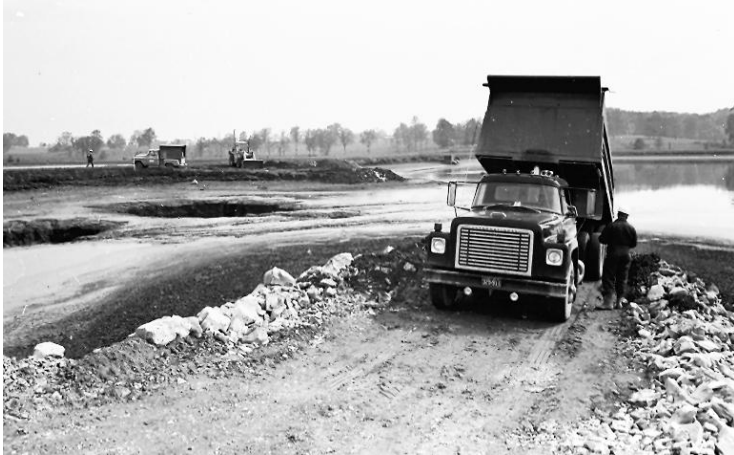
Above: Haulers dump rock to build a dike to isolate sinkholes on left. (Photo courtesy West Plains Daily Quill)
